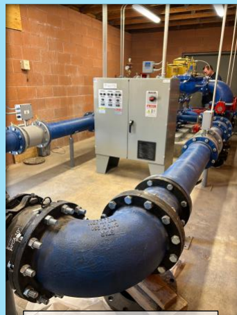
Vista Del Monte Booster Station
